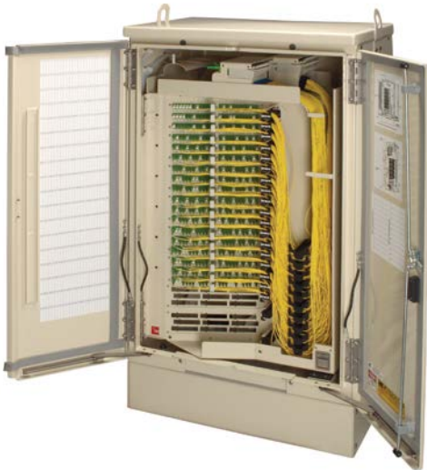
Figure 2: Fiber Distribution Hub
