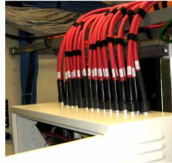
Interlocking armor fiber cables installed in cabinet
