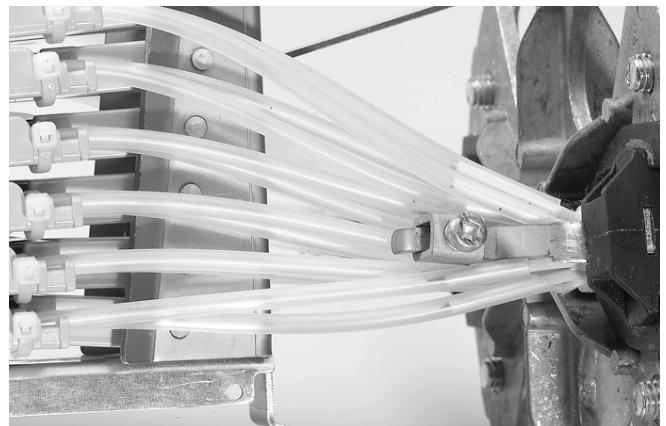
6.1.4 Cable installed with single bracketlet.
