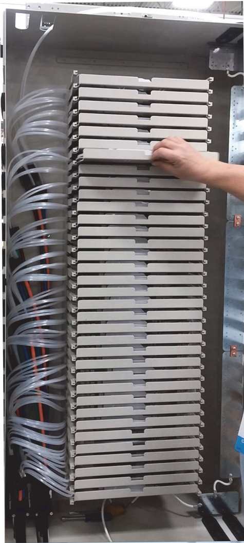
Figure 21. 10K Fiber Entrance Cabinet (FEC) With Compact Interior Drawers for Splices
